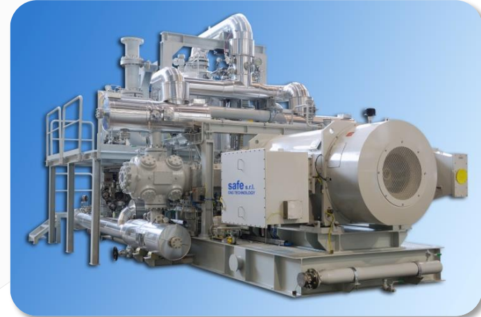
KUWAIT – FUEL GAS BOOSTER SKID
