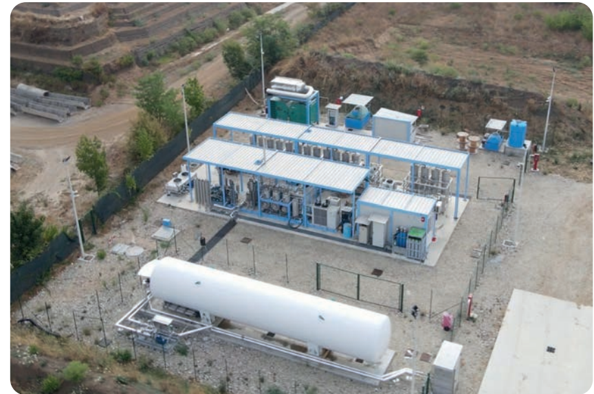
Novi Ligure - Landfill managed by SRT S.p.A Biogas upgrading + biomethane liquefaction & storage
